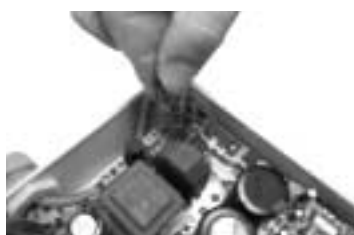
Motor cables on the inverter
